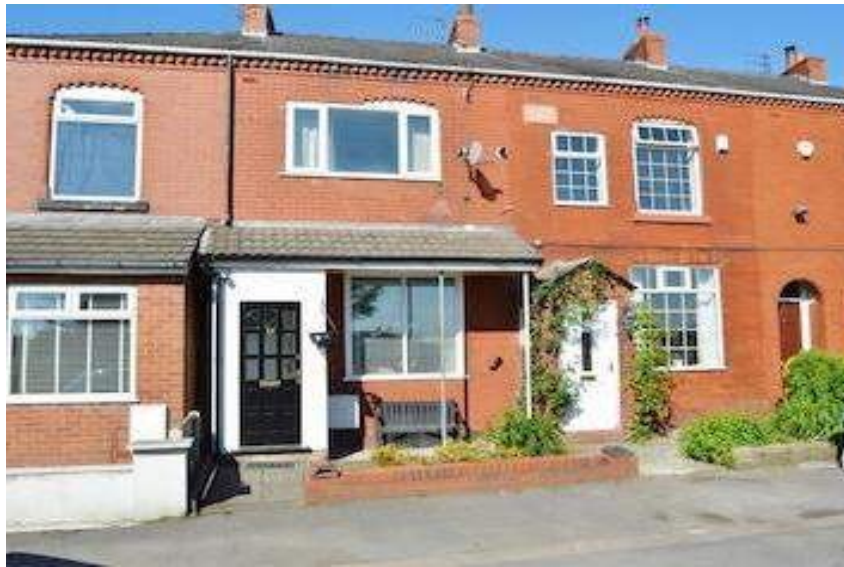
A row of cottages with some of the most appalling disfigurements imaginable.
